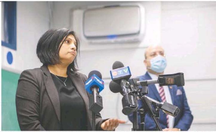
Tanya Alvarez, principal at Pierre Elliott Trudeau Elementary School in Rosemont, and EMSB chairman Joe Ortona stand in front of a newly installed air purifier at the school on Monday. The school is one of 30 buildings the board is in the process of equipping with the devices. DAVE SIDAWAY
